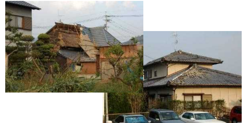
Figure 1 Structural damage due to Typhoon Tokage (0423)
