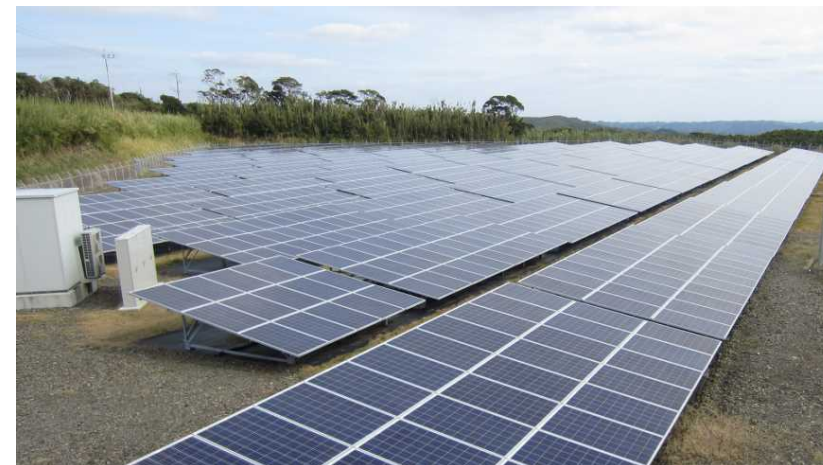
Figure 1 Photovoltaic system in a island
