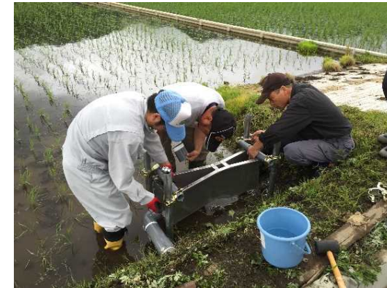
Figure 1 水文計測装置の現場設置 Set up of a hydrological measurement instrument
