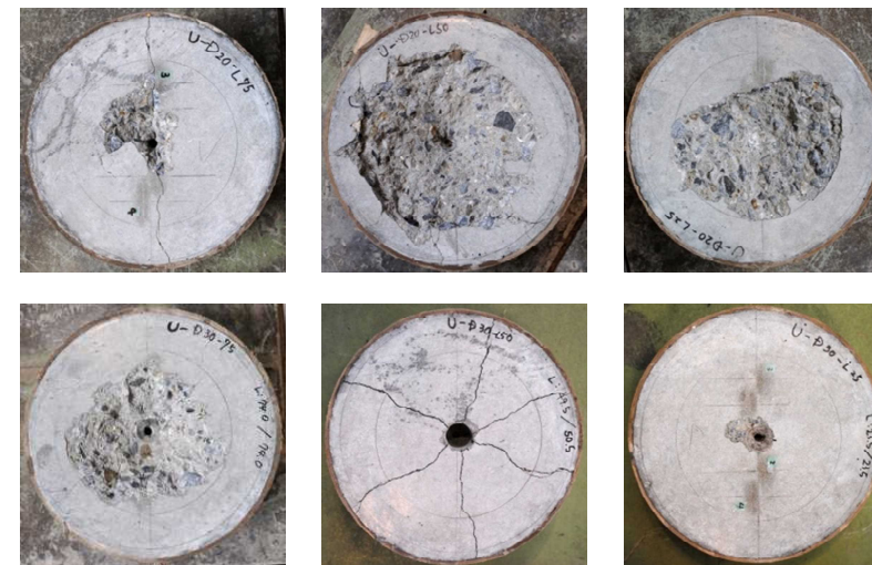
Figure 1. Crack pattern of post installed adhesive anchor.
