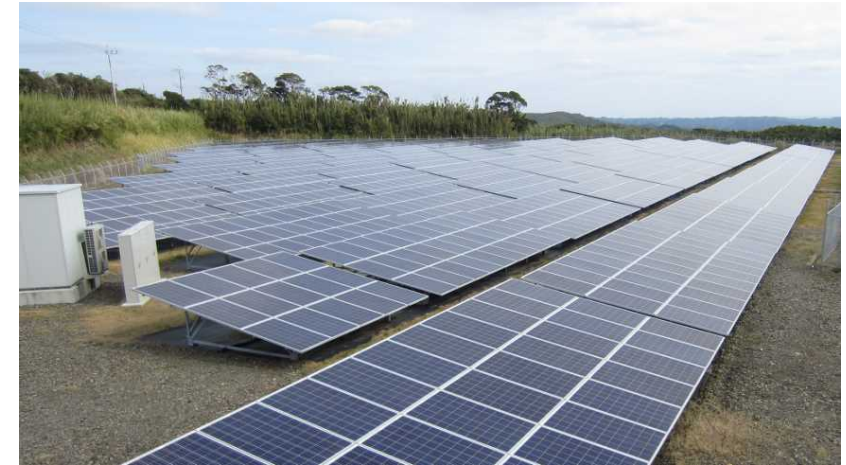
Figure 1 Photovoltaic system in a island
